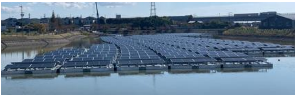
▲Floating solar panel arrangement
