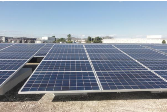
▲Solar panels at the Iho Site,
