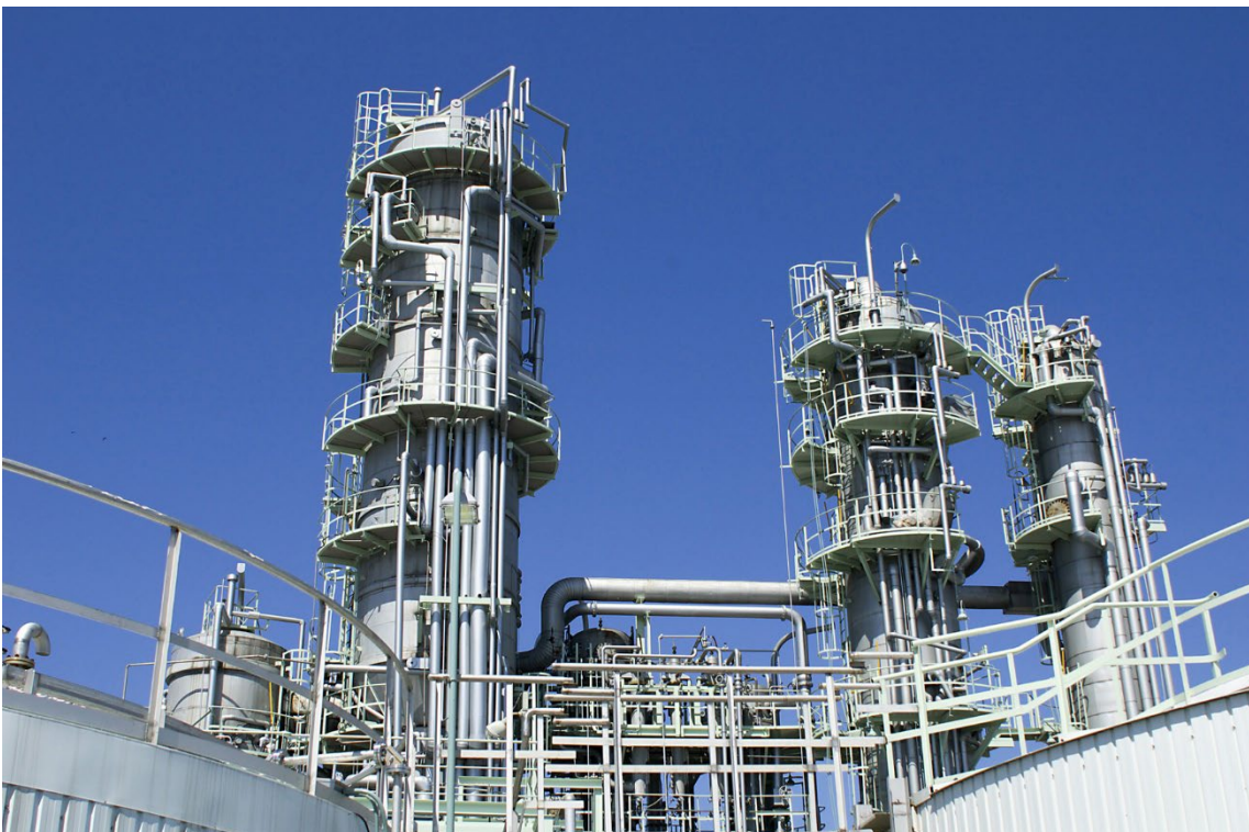
Tall Oil Distillation Plant (As of 2025)
