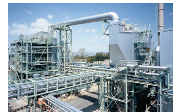
Biomass Power Plant
