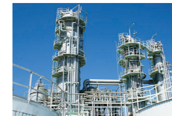
Tall Oil Distillation Plant
